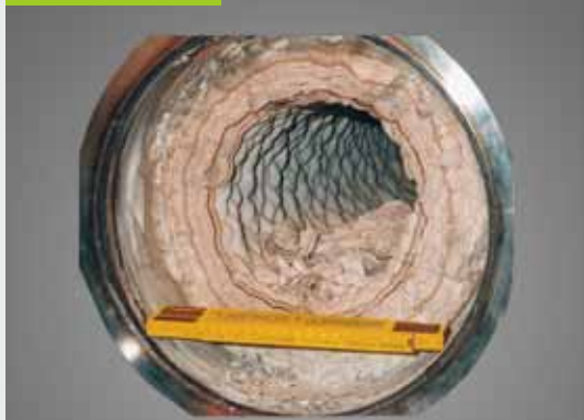
Pipe Before Cleaning
